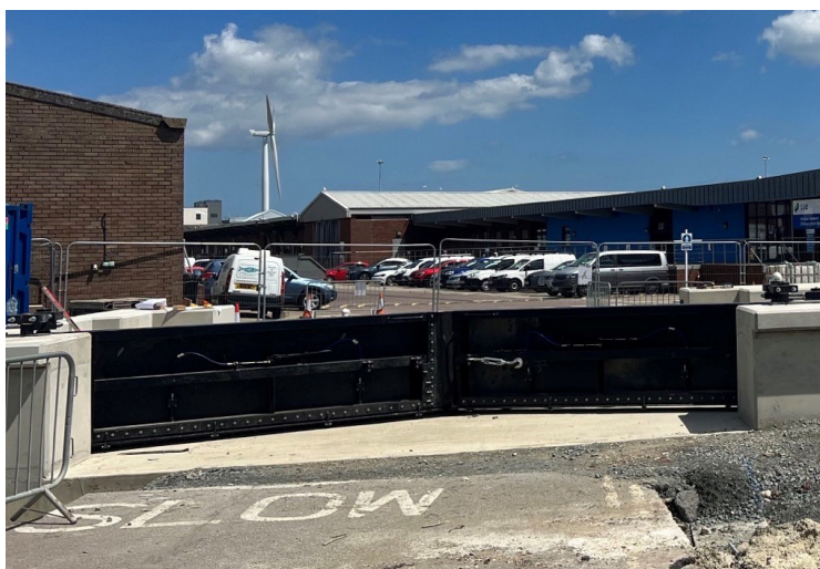
Flood gates installed in the port entrance.
