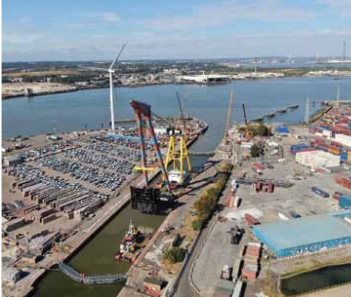
Replacement mitre gate being brought into the Port of Tilbury lock for installation as part of the Tilbury Barrier replacement works
